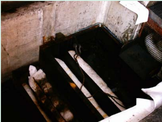
Oil water separator
