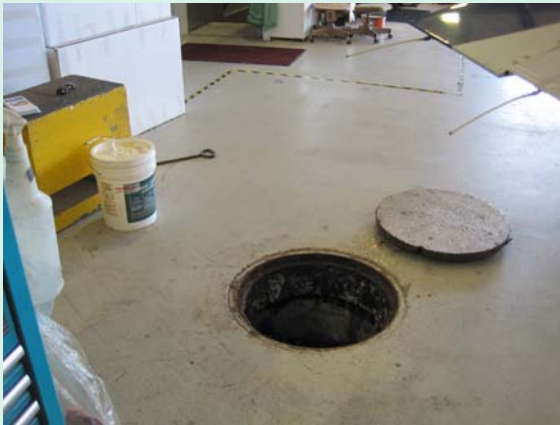
Oil water separator in maintenance hangars
